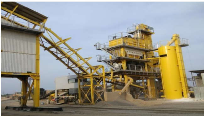
Bitumen and concrete hot-mix plants at the project sites
